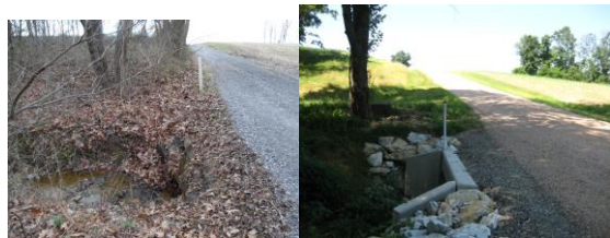
Culvert crossing replaced on Bittle Road, Germany Twp from a 30 inch pipe to 9 foot wide box culvert
